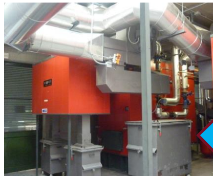
Chipped wood boilers
